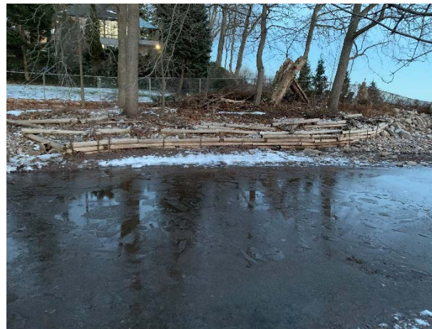
Photo F – Failing Crib Wall Erosion Protection Measure at the Confluence with Lake Ontario.
