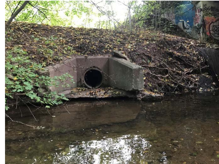
Photo A – Undermined Storm Outfall Upstream of Lakeshore Road.
