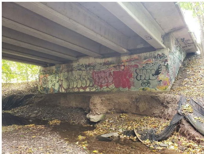
Photo B – Failed Bridge Abutment Protection at Lakeshore Road Crossing.
