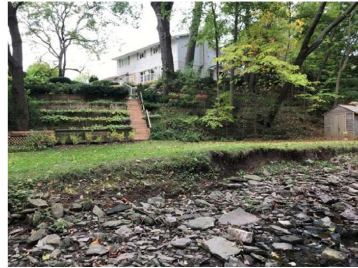
Photo D – Manicured Lawn on Private Property Experiencing Eroding Riprap Application.
