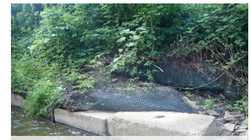
AOC 3 - failing erosion control
