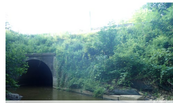
AOC 3 - armourstone slope protection is outflanked
