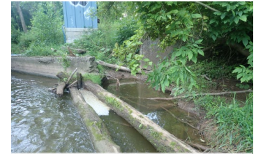
AOC 4 - failing bank protection
