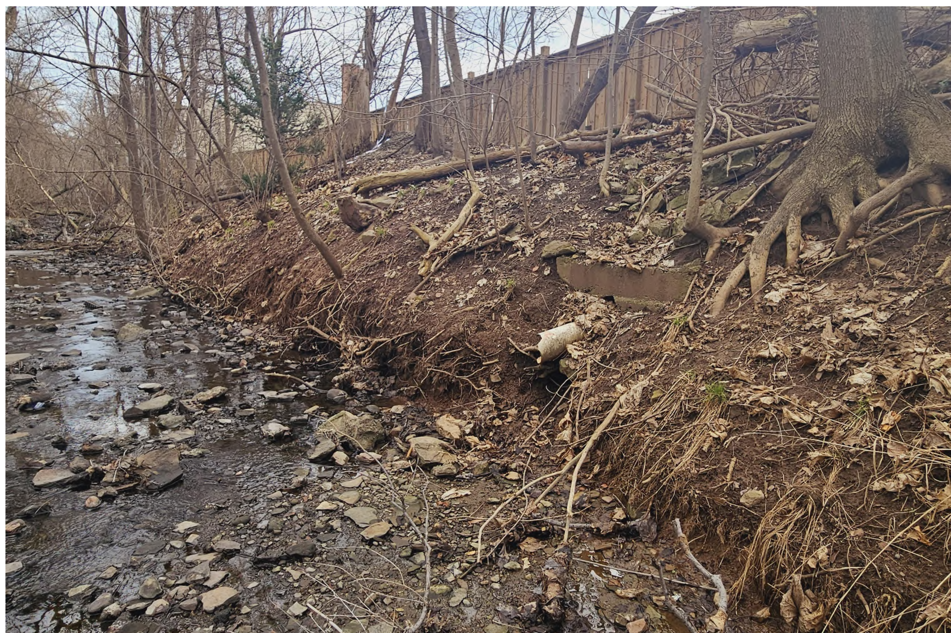
Photo B – Active Erosion Along the Toe of the Bank and Deteriorated Storm Outfall
