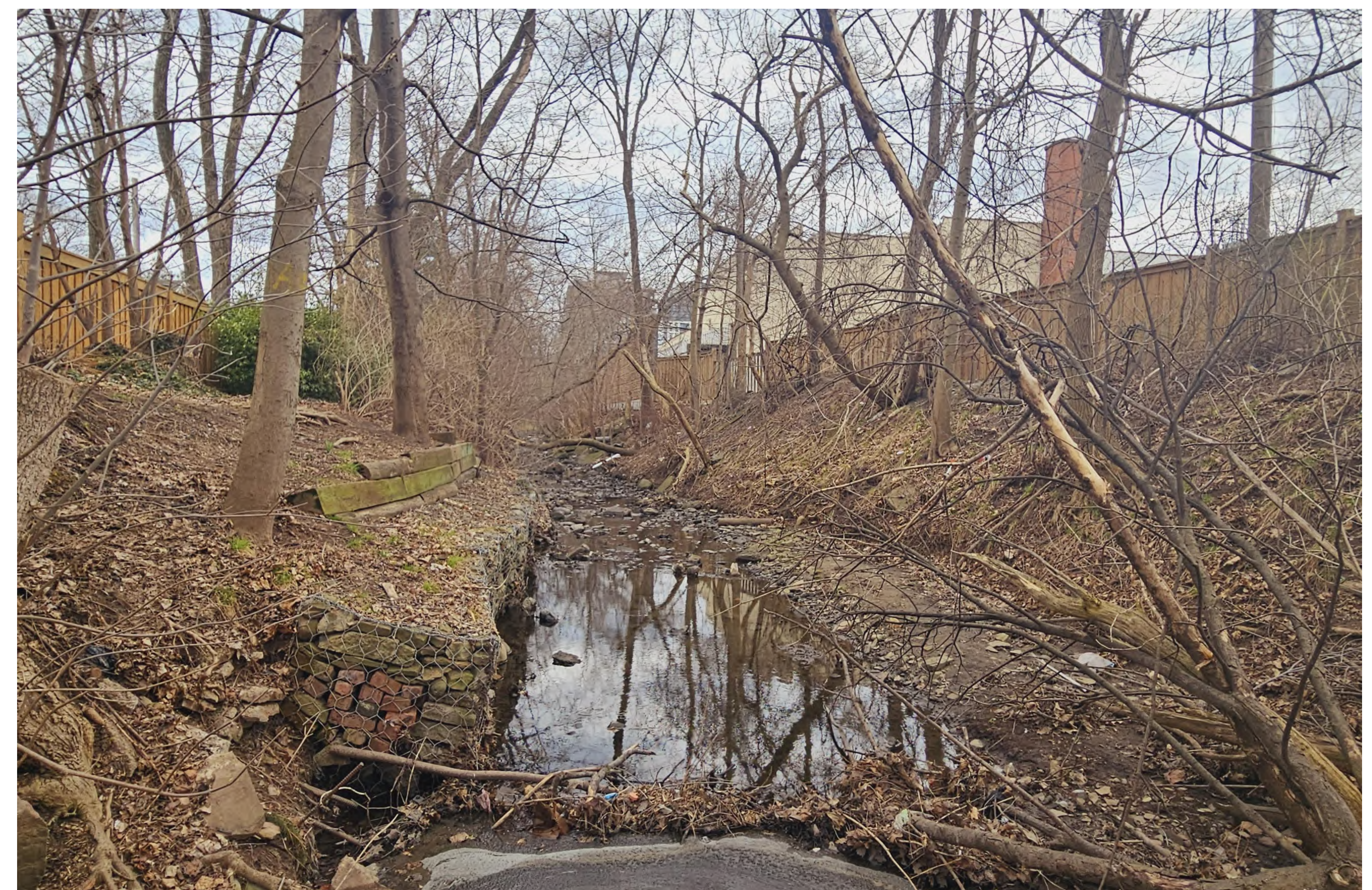
Photo C – Leaning Gabion Baskets and Timber Retaining Wall
