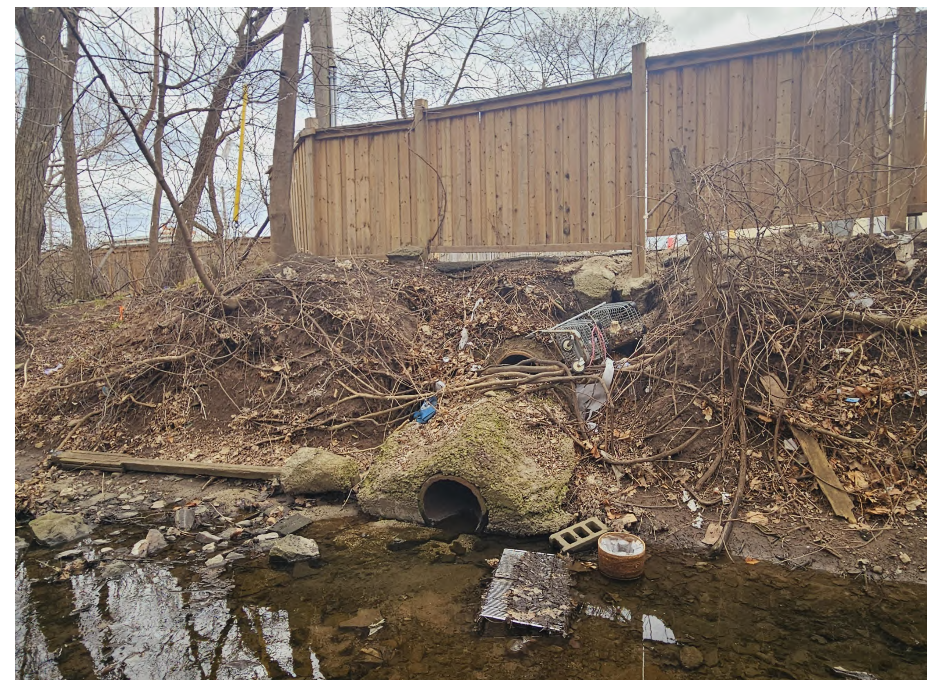
Photo D – Broken Storm Outfall Along the West Bank and Exposed Fence Concrete Footing
