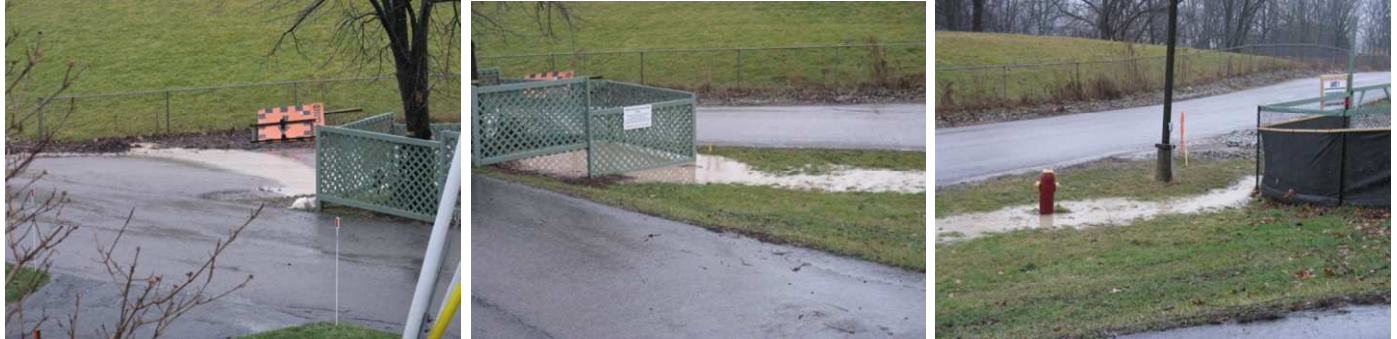
Jan. 13, 2013 –Junction of Residential Access Laneway and CAMA Woodlands Perimeter Road with surface runoff from the construction site. The sloping topography NW of Craven Avenue could flood Nevarc Drive and adjacent properties.
